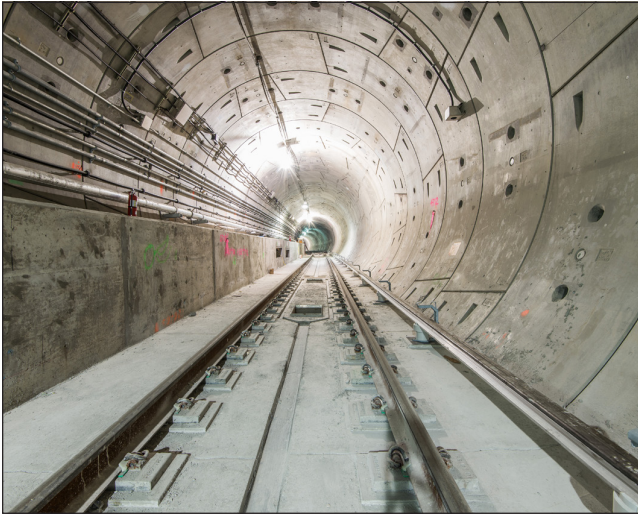
↑ $2.7B East Side Access (multiple projects), New York ↓ New York Metropolitan Transportation Authority
