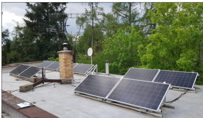
Figure 4: Installed solar panels on the roof of the house
