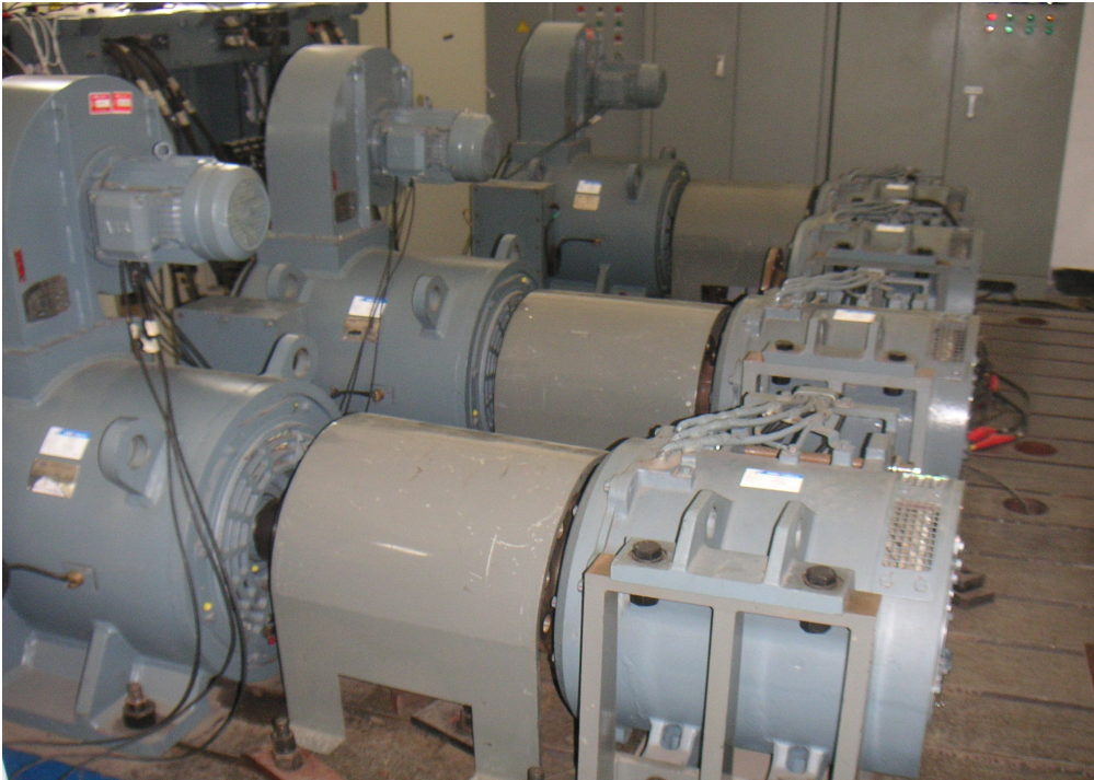
Fig. 59: Right: YJ150B 180kW induction machines on a test bench stand; Left: load machines YJ209A.
