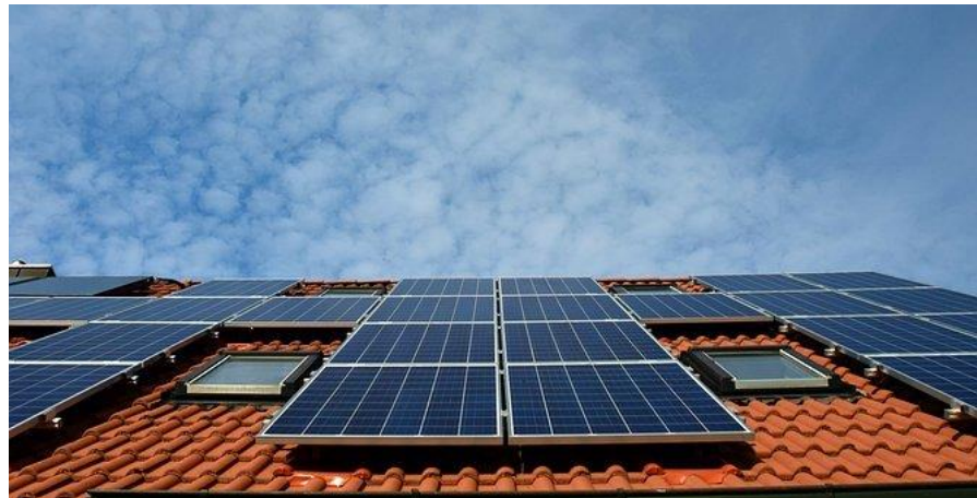
Figure 3: Photovoltaic Cells on the roof of a house (Pixabay Stock Image).
