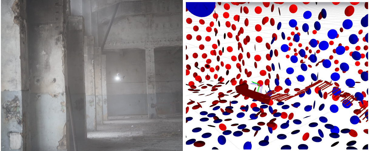
Figure 7.11: The UAV inspecting surfaces on the wall of the brewery's upper room both on camera (left) and at approximately the same time in RVIZ (right)
