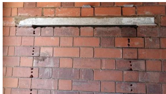
(Photo. 46. Insolation of lintel from one side.)
