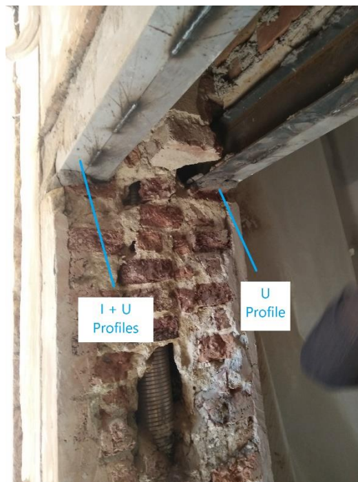
(Photo. 28. Failure of installation of Lintels.)
