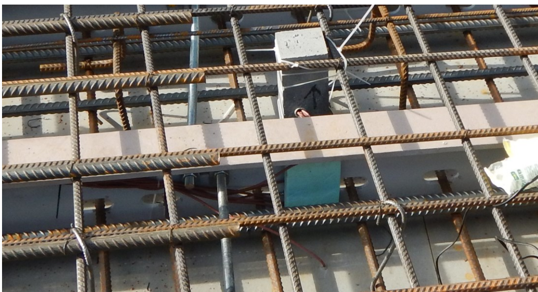
Figure 56 Bunch of thermometers on filler beam, covered by XPS insulation. Casing beam is behind the filler beam. (picture: J. Zatloukalová)
