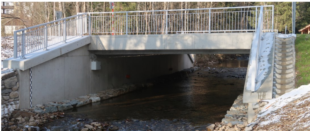
Figure 59 Bridge No. 27-117 with installed switchboard box on the left abutment (picture: J. Zatloukal)
