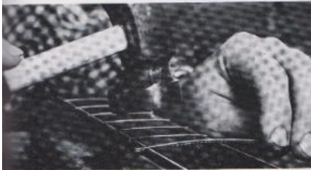
12-23. Driving in the fret from one end to the other. The first blow must keep the fret vertical.
