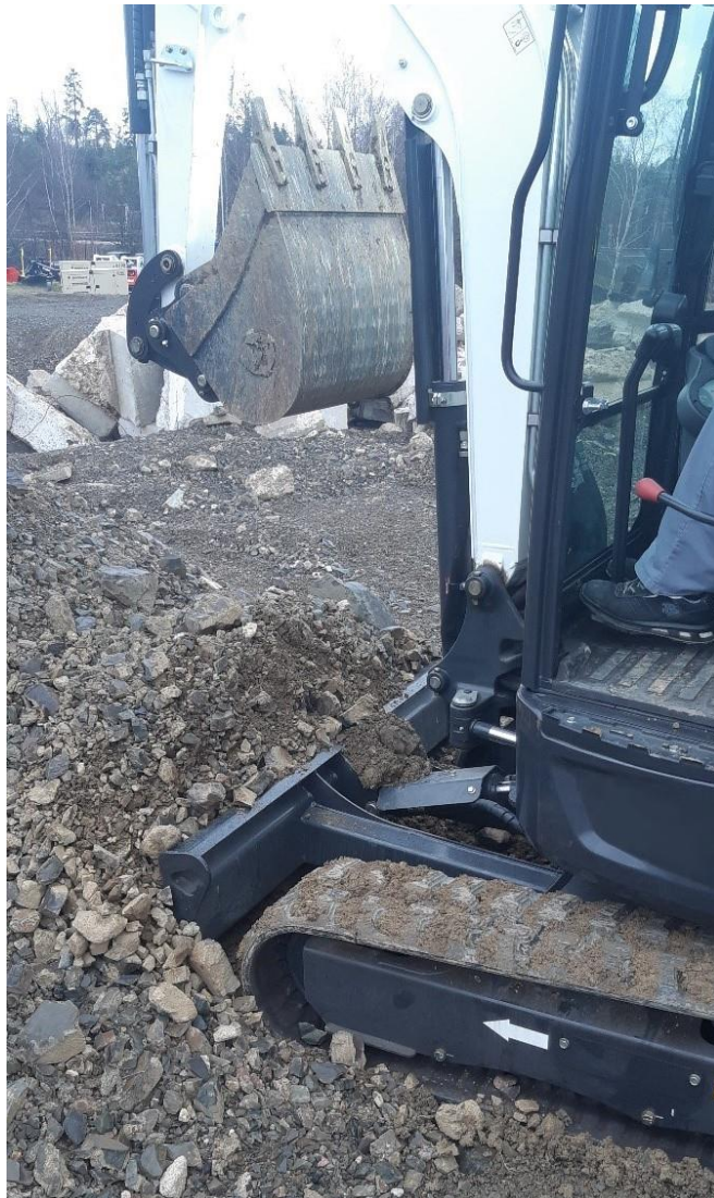
Figure 77 Excavator is pushing into a pile of dirt to overload the engine
