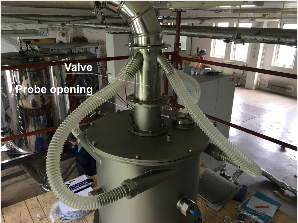
Figure 8.7: Location of the valve and anemometer probe
