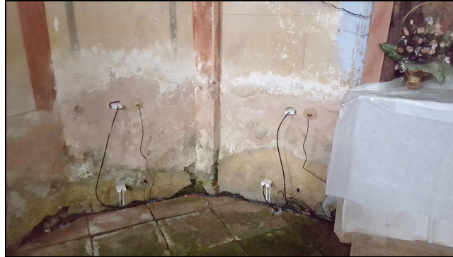
Figure 25 Inside measurement station in St. Anna church
