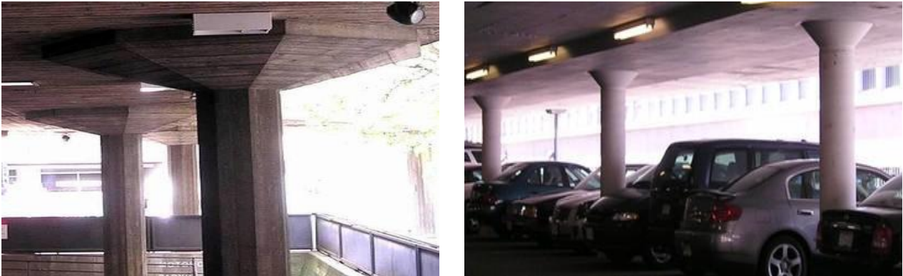
Figure 3: Reinforced concrete flat slab with a column capital, London, UK (left) and concrete flat slab with head, Vancouver, Canada (right)
