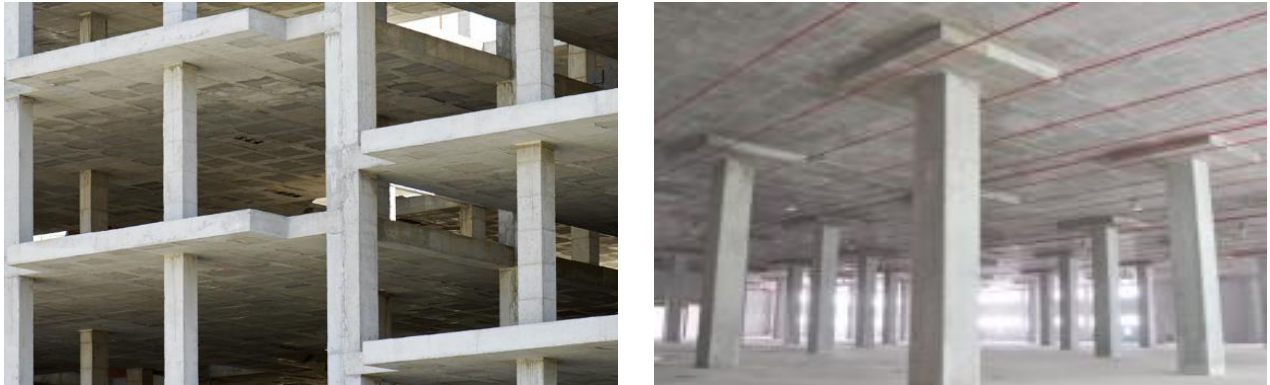
Figure 1: Flat slab without drop and column head (left) and flat slab with drops (right)
