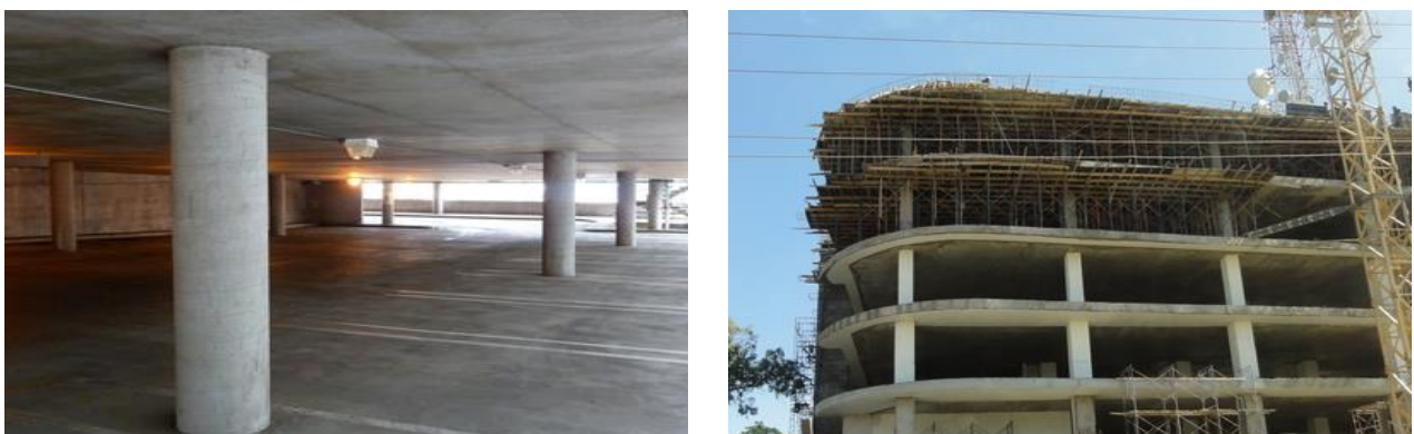
Figure 2: Reinforced concrete flat plate system, Eugene, USA, (left) and a reinforced concrete building with flat plate system under construction, Kenya (right)
