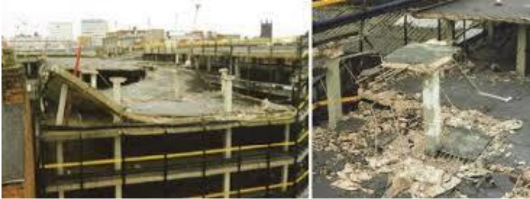
Figure 7: Upper floor collapse of Wolverhampton parking (UK)
