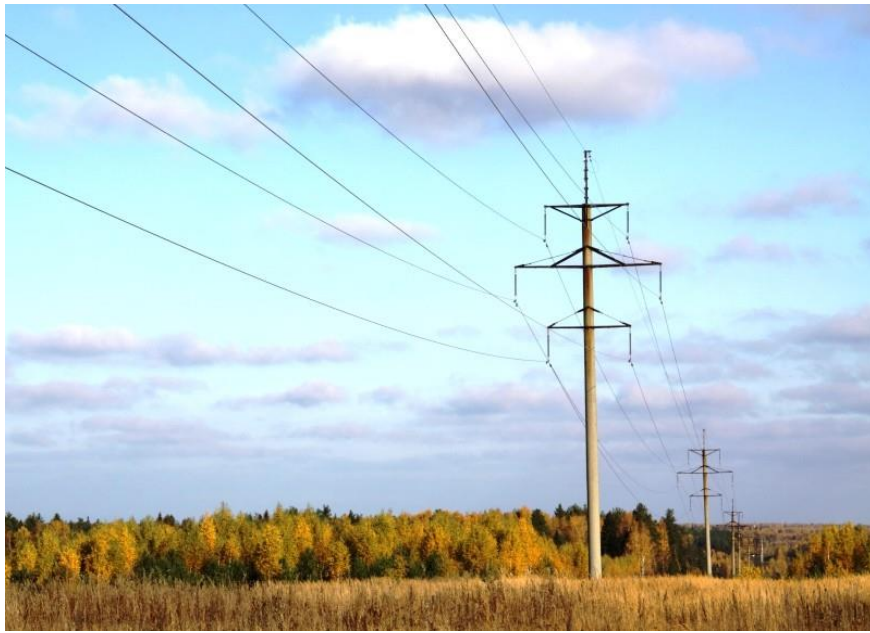
Figure 3 – Overhead transmission power line. [5]
