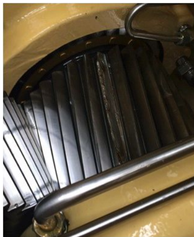
(c) a photo of the fault
