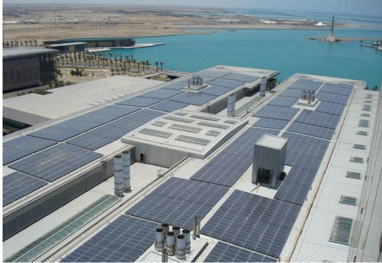
Figure 3.5: The 2 MW rooftop solar plant at KAUST [7]
