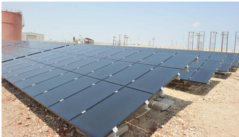
Figure 3.6: Solar power plant on Farasan Island, Southwest Saudi Arabia [7]
