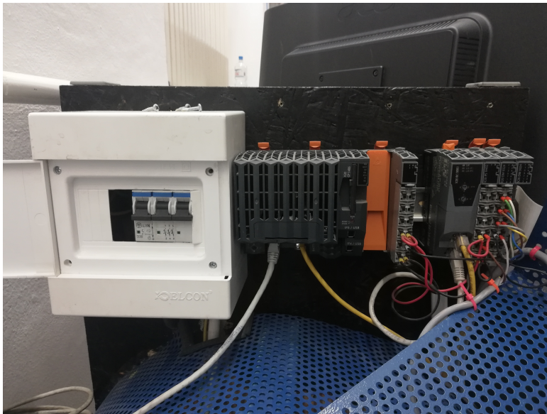
Figure 3.3: PLC unit on the right, circuit breakers on the left
