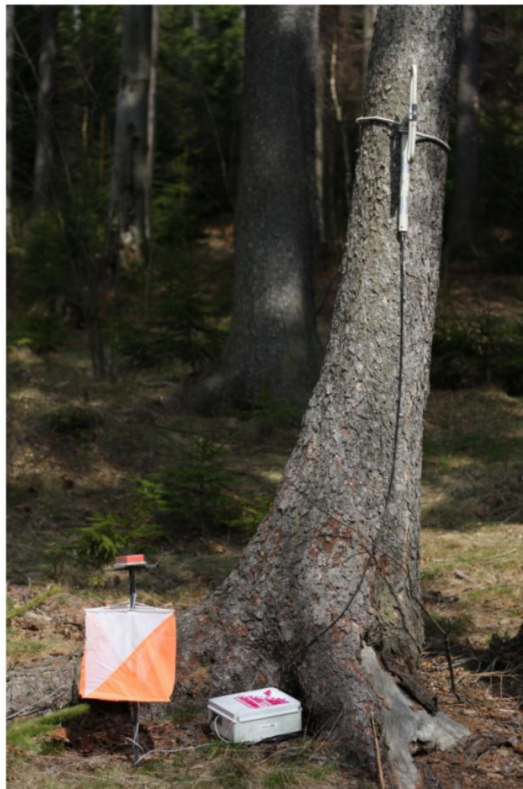
Figure 4.10: Racom device with the external antenna mounted on a tree. Source: [Rac20]
