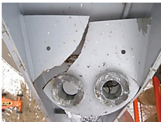
Fig. 3. Failure of cable anchorage due to fatigue cracking as a result of vortex excitation at the Martin Olav Sabo Pedestrian Bridge in Minneapolis, USA (Santosuosso et al., 2012).
