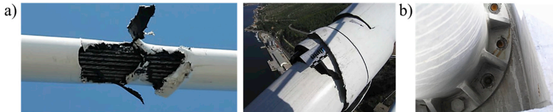
Fig. 2. Example of damage to (a) bridge cable cover sheath and (b) cable anchor resulting from cable icing conditions and wind action at the Dubrovnik Bridge, Croatia (Savor et al., 2006).
