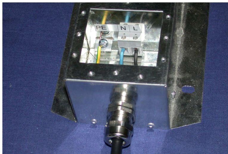
Figure 4.9: Opened box with PE, L and N terminals and connected power-line cable wires.
