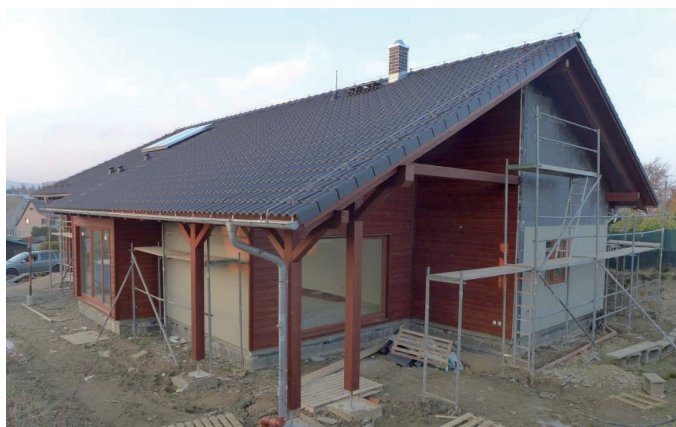
Fig. 4 Building 4 – The family house in Rýmařov (source: Kabele, Urban: Grant no: te02000077 Smart Regions – buildings and settlements information modelling, technology and infrastructure for sustainable development)
