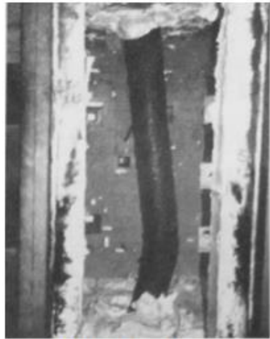
b) Overall buckling
