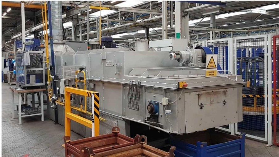
Figure 13: Continuous gas dual-zone furnace Ipsen
