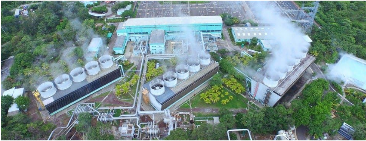
Figure 1.5.3 Berlin geothermal power plant of La Geo in El Salvador (binary cycle)
