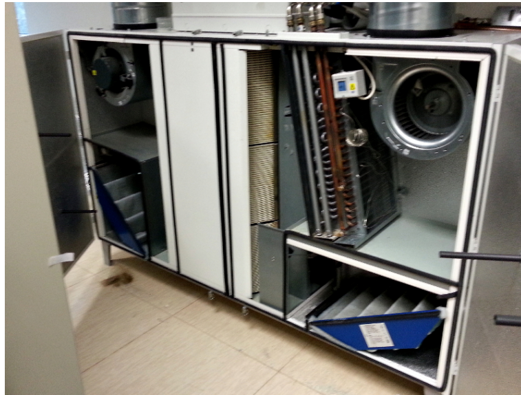
Figure 5.8: General view of an open AHU
