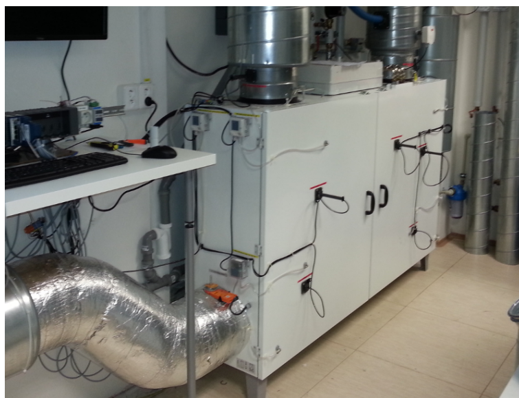
Figure 5.7: General view of AHU with new sensors
