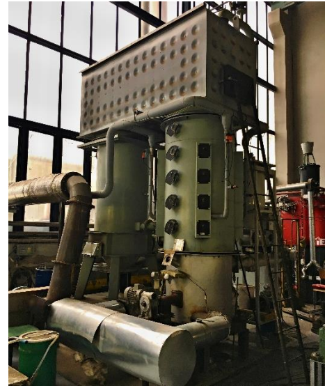
Figure 6-5: Photograph of the FBC boiler Golem
