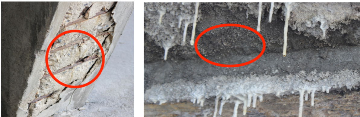
Figure 88 – Rock pockets in a concrete column.
