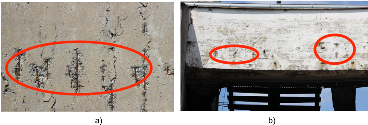
Figure 83 – Non-connected cracks: a) regular distance; b) irregular distance.
