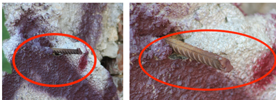
Figure 86 – Chromatic alteration in concrete wall.
