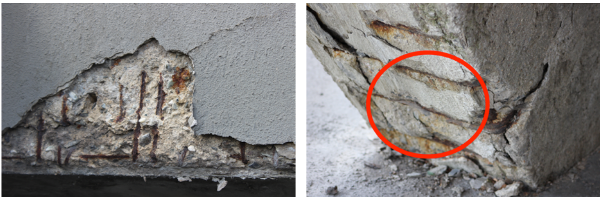
Figure 94 – Pitting reinforcement corrosion in North tribune.
