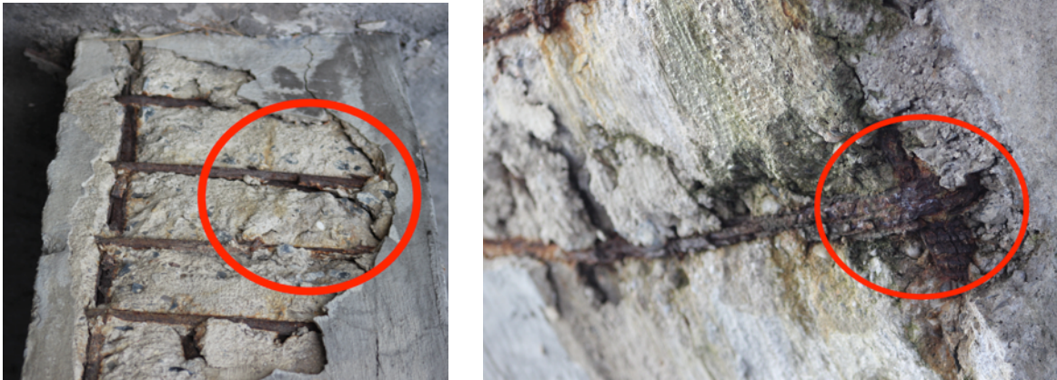
Figure 95 – Loss of rebar diameter in column of North tribune.
