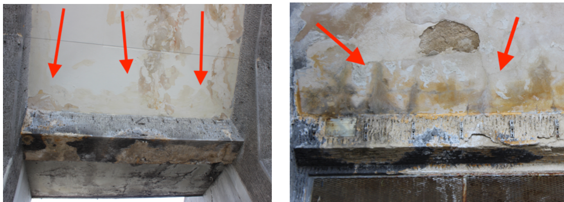
Figure 93 – Bending in the junction of beams and slabs.
