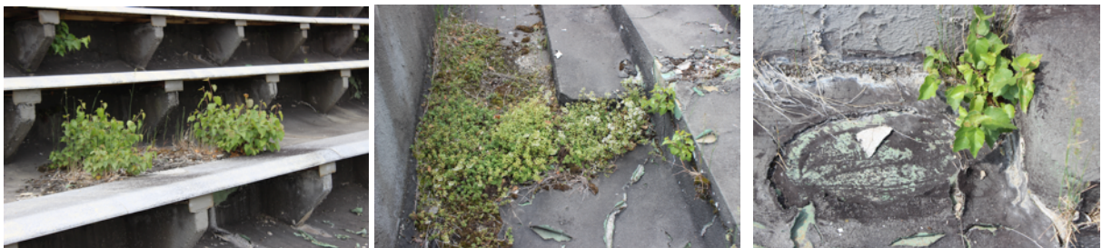
Figure 90 – Higher plants on the grandstands of North tribune.
