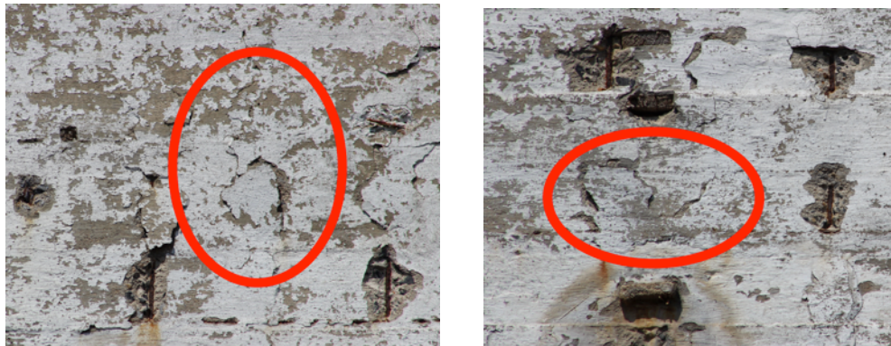
Figure 85 – Map-cracking in North tribune.
