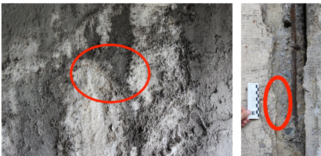
Figure 80 – Scaling in North tribune.
