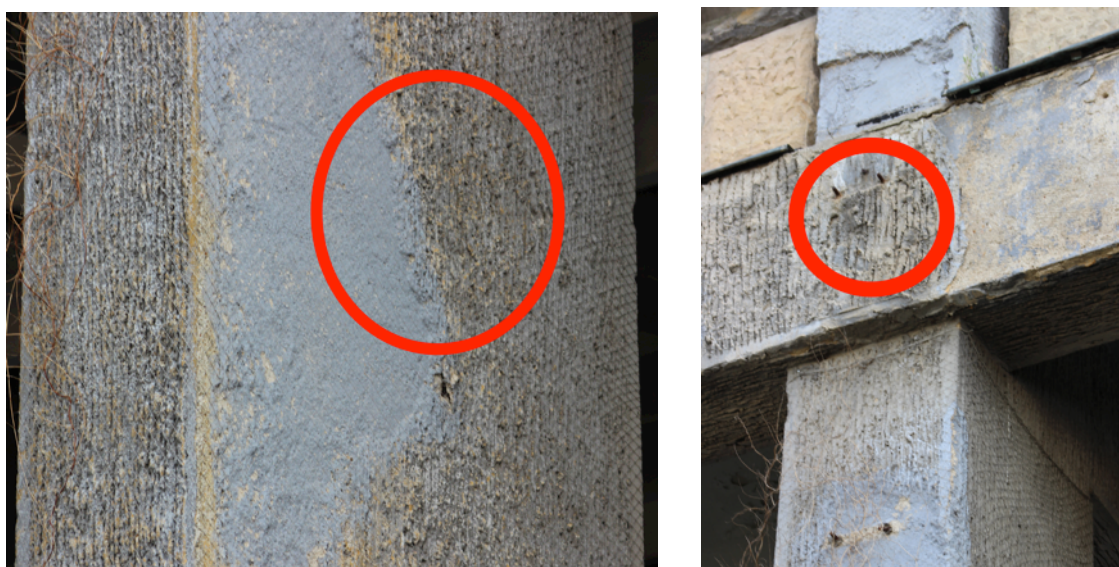
Figure 82 – Exfoliation in the column in North tribune.
