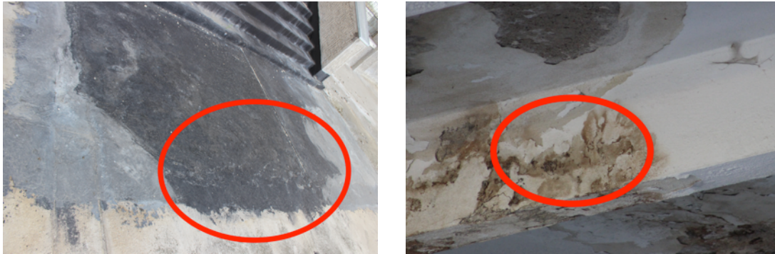
Figure 87 – Moist spots in a concrete wall.
