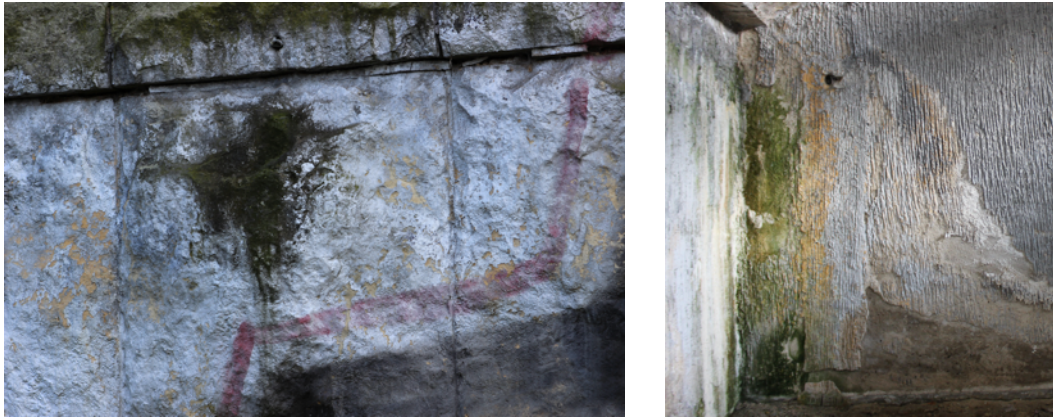
Figure 92 – Algae presence on concrete walls of North tribune.
