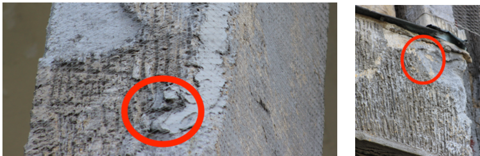
Figure 77 – Concrete erosion in North tribune.
