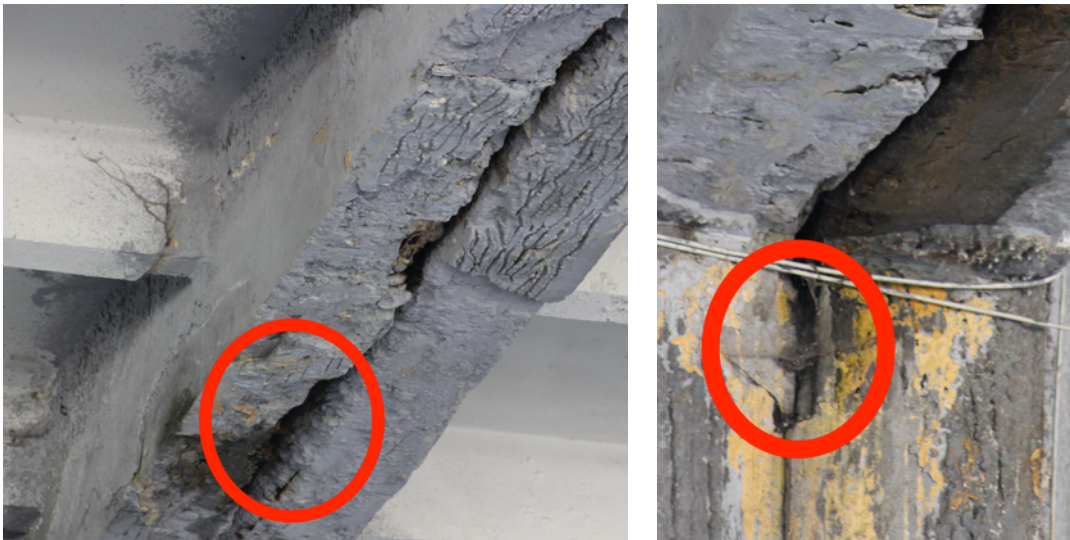
Figure 81 – Spalling occurrence in North tribune.
