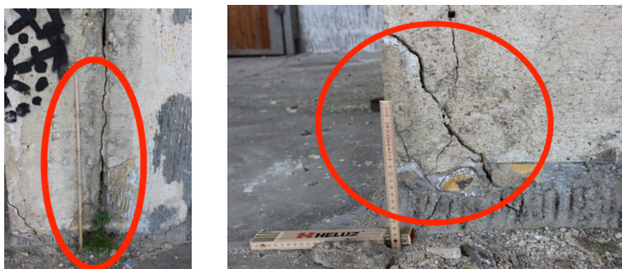
Figure 84 – Individual cracks in North tribune corridor.
