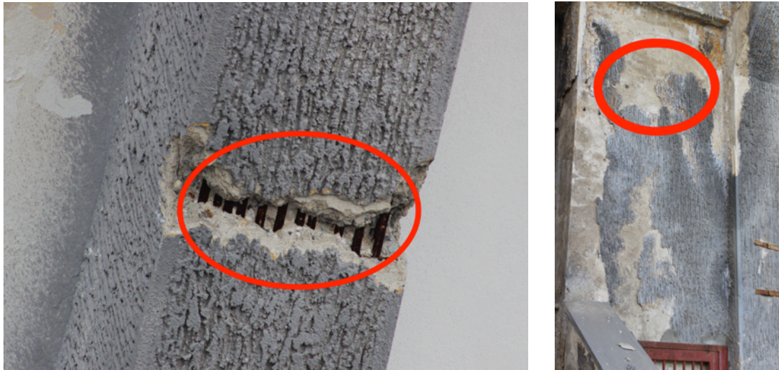
Figure 79 – Crumbling in North tribune.
