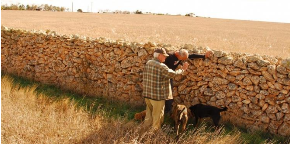
Figure 16 Edithburgh dry masonry wall [9]
