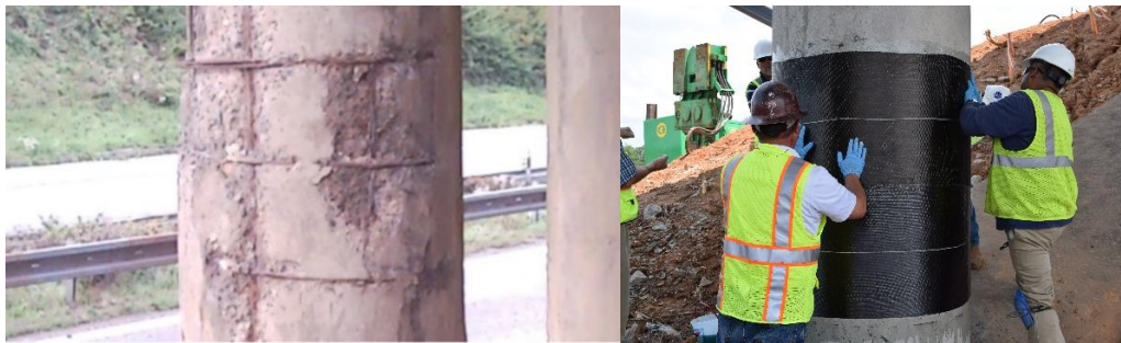
(Fig. 7: Damaged pillar of the bridge. Source: Roads & Bridges, 2019).
