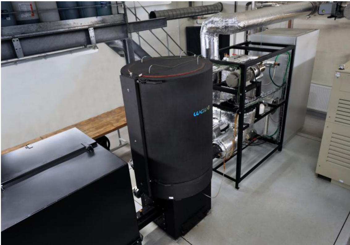
Figure 2.2: A picture of the 50 kW ORC unit, Wave 50 in laboratories of UCEEB, CTU [40]
