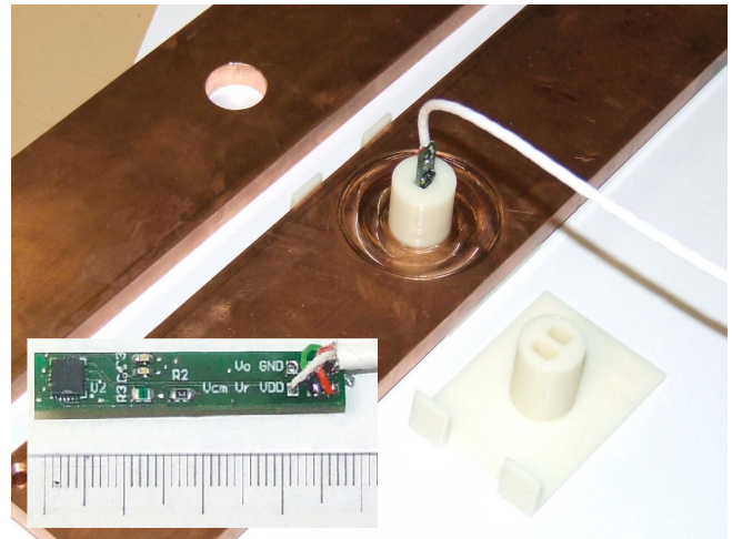
Fig. 6. Basic busbar sensor and amphitheater busbar current sensor with two sensors in the holder. Inset: Printed-circuit board (PCB) with fluxgate sensor.
