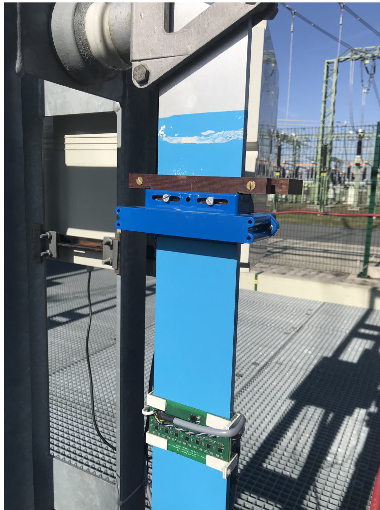
Figure 7.1: Installed rectangular and LEM current sensor on the neutral line in Mírovka distribution station
