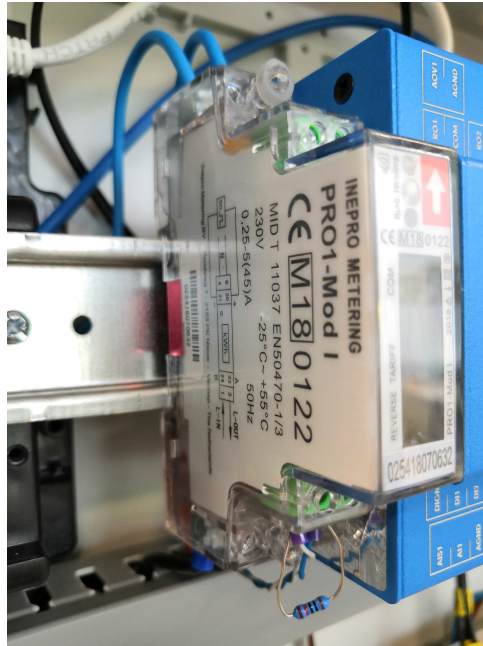
Figure 2.12: PRO1-Mod electricity meter
