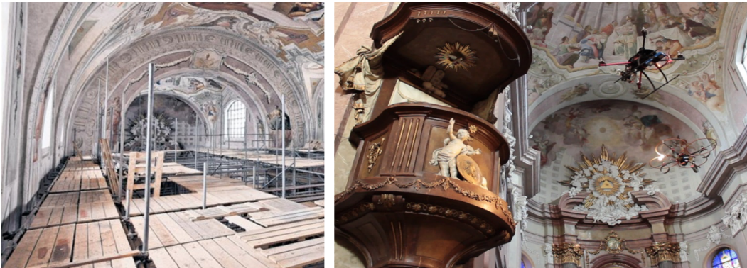
Figure 16: The motivation for using MAVs in the inspection task in the interiors of historical objects. Left: Scaffolding in the church in Šternberk required for manual inspection. The church was closed for four months for services and tourists. Right: The same work in the same church conducted by our MAVs eight years later. The church was closed for four hours only.
