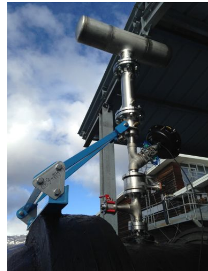
Figure 1.10: Photo of degassing system installed on the Thermosiphon condenser
