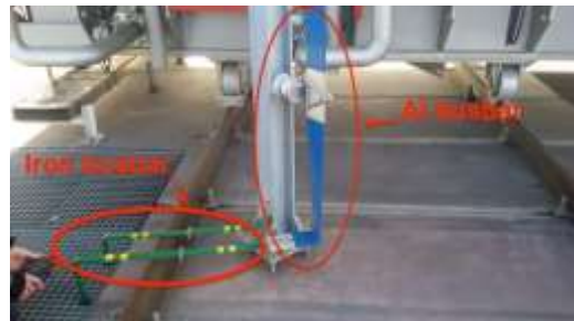
Figure 1: Al and Iron busbar as a ground conductor at the power station in the Czech Republic
