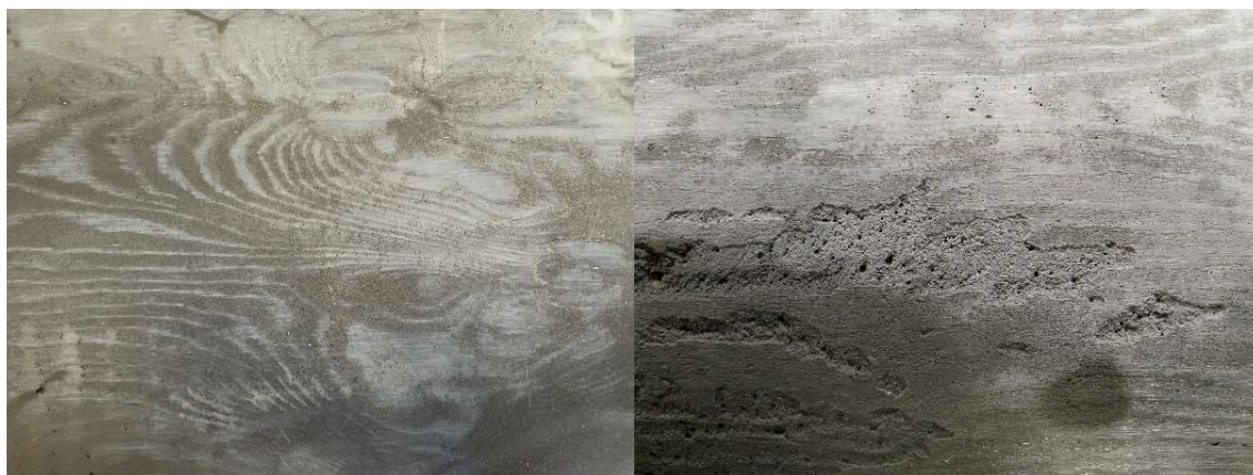
Obr. 72: Detail textury, defektu
