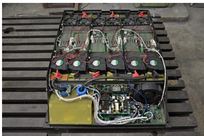
Figure 29 Battery of FSE.06 [21]
