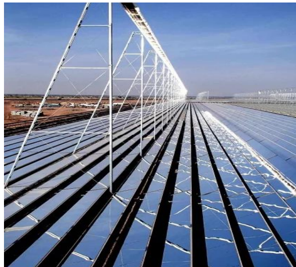
Fig. 3.10. Dhursar Fresnel reflector solar power plant [16].
