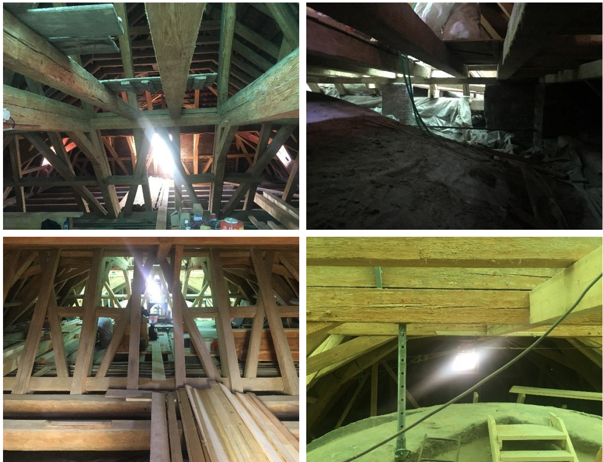
Figure 3.15 – The western part of the church’s roof (top-left), the wall openings of the older church (top-right), the central roof of the church (bottom-left) and the eastern part of the roof (bottom-right)
