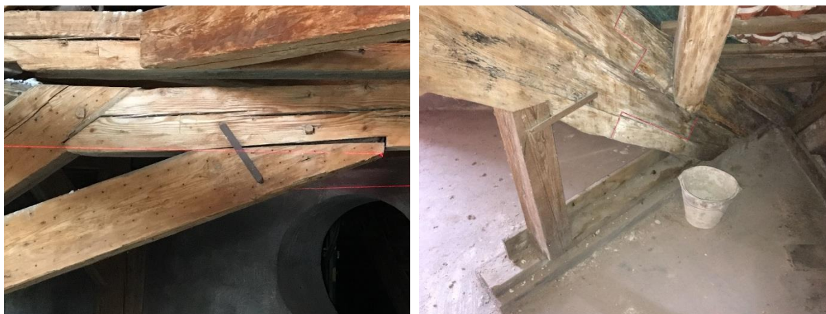
Figure 3.21 – The metallic element in the diagonal strut (left) and the prosthesis (right)
