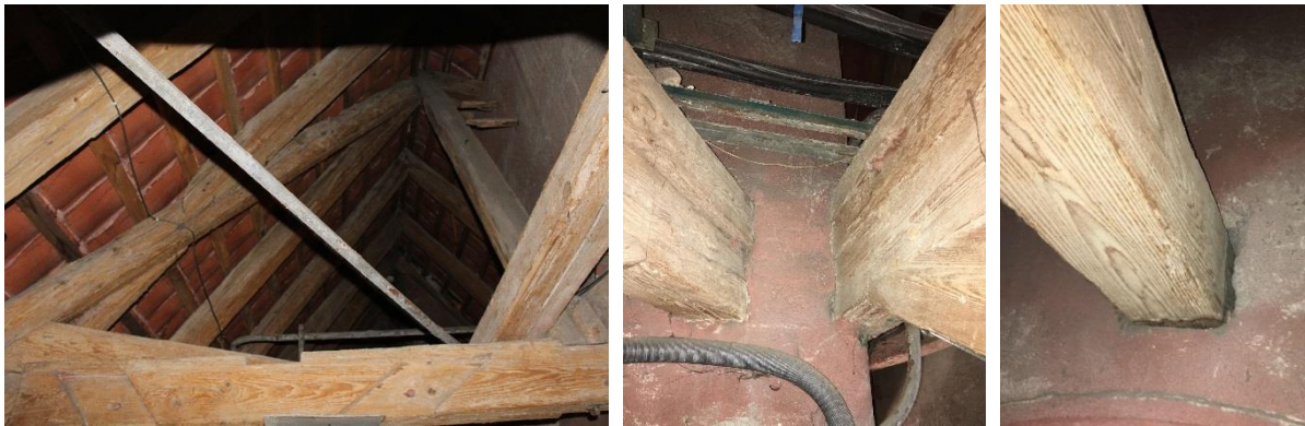
Figure 3.14 – The base plan of the southern part of the west wing roof (top), the traces of the original roof (left), the original tie beam (center) and the new tie beam (right)
