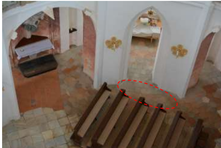
Figure 12- Lighter shade of tiles observed cause by heavy traffic and abrasion.
