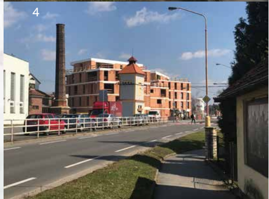
4 new residential complex with commercial units in parterre in construction, originally slaughterhouse at this place
