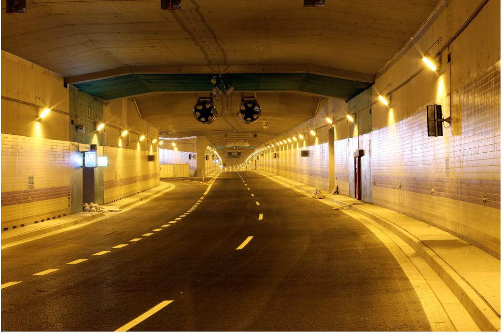
Figure 2.1: On the left, the entrance ramp Prašný most can be seen. Additionally, a pair of jet fans is located at the ceiling of the tunnel.
