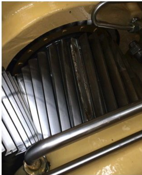
Figure 5.7: A fault found on the wind turbine gear, source: [4]
