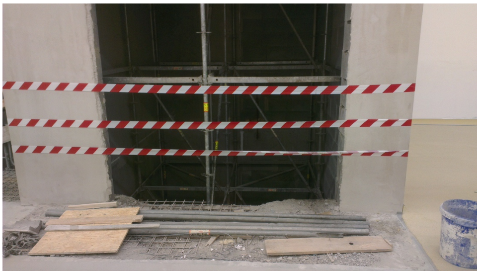
Picture 19 - poor security of the elevator shaft
