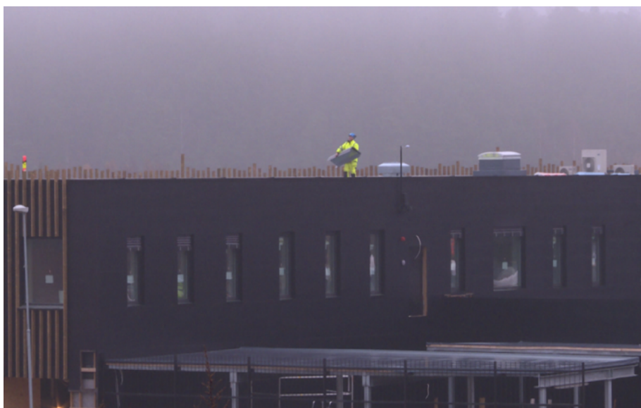
Picture 8 - worker walking on the roof without security against the fall
