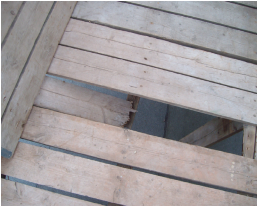
Picture 4 - broken floor of scaffolding
