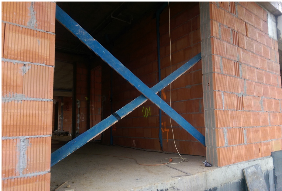
Picture 12 - poor protection of edge with risk of fall
