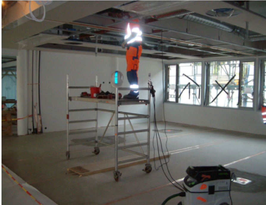
Picture 9 – poor security of work in height
