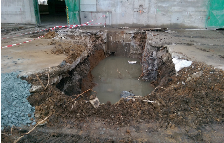
Picture 14 - unsecured building pit
