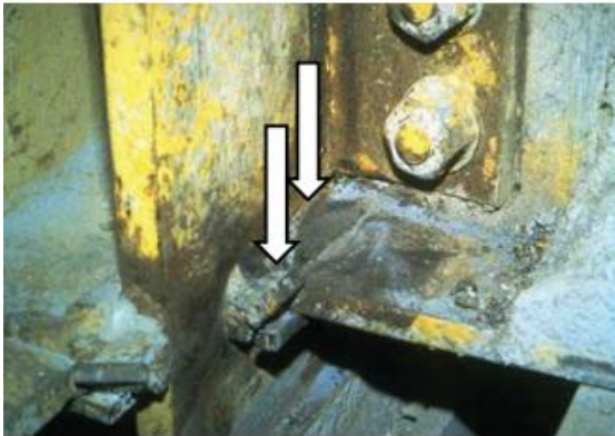
a) Fracture of beam flange at JP groove weld.
