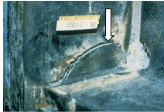
b) Fracture involving divot of steel.
