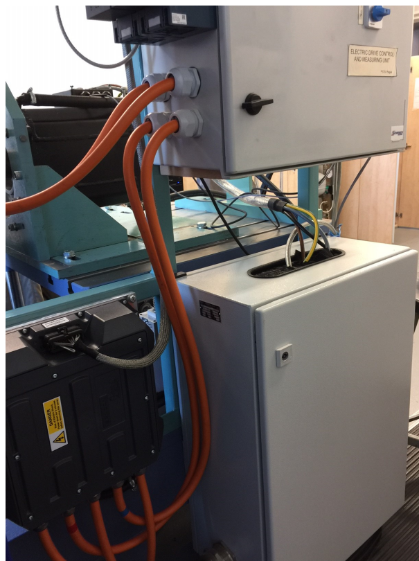
Figure 5.12. Sevcon power converter with control and measurement unit
