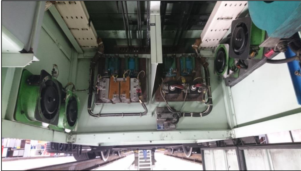
Figure 20: Picture of the box with ventilation and diodes
