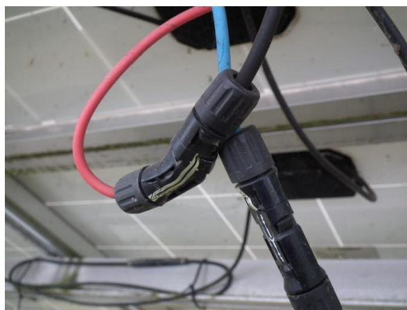
Fig. 20: Thermally damaged connector
