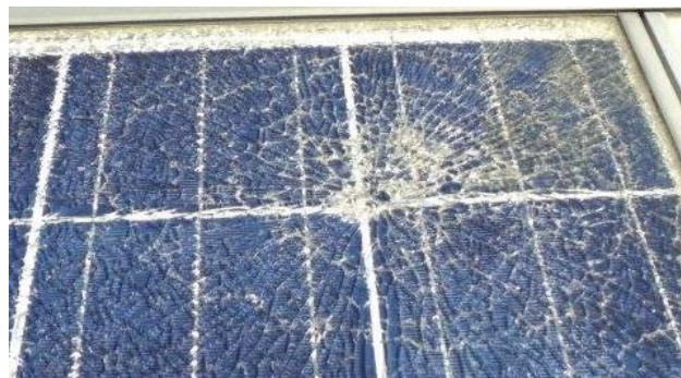
Fig. 18: Front glass damage caused by a stone
