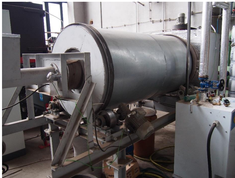
Figure 5.1 Steam drum dryer, CTU laboratories
