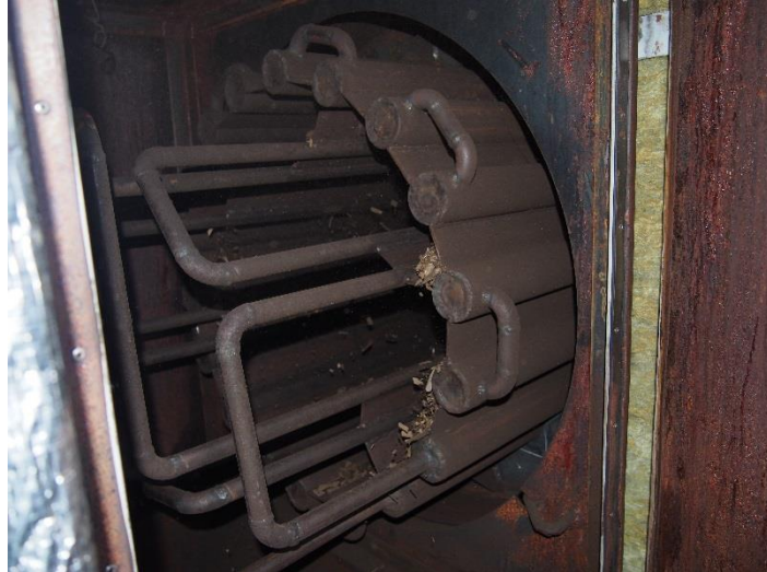
Figure 5.5 View of the drying chamber
