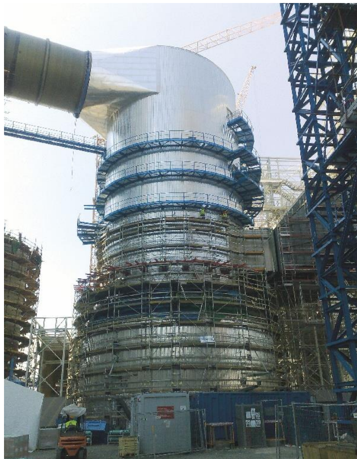
Figure 10- The FGD unit before completion in Ledvice [44]
