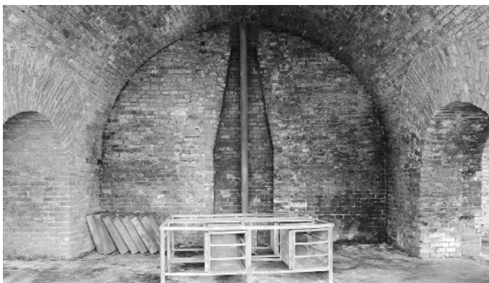
prosotry pod valem (bastion 1)
